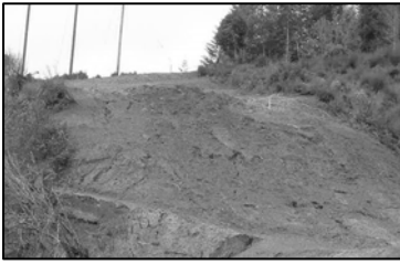
Numerous landslides and massive erosion was caused by the 2004 pipeline project near Coos Bay
